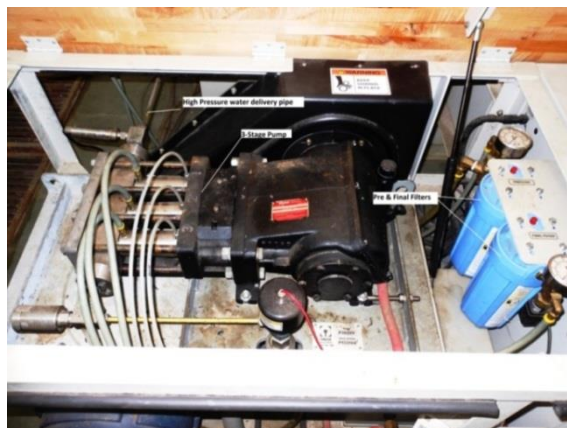
Fig 3.2: High pressure generation pumping system
